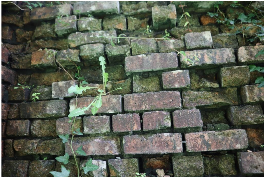
Figure 4.17. Frost damaged bricks
