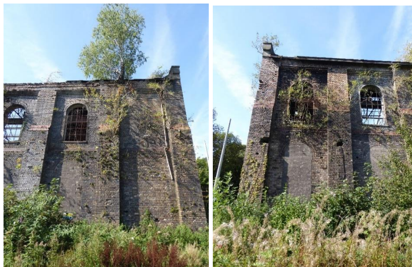
Figures 13 to 15 Images showing condition of roof and extent of vegetation to brickwork
